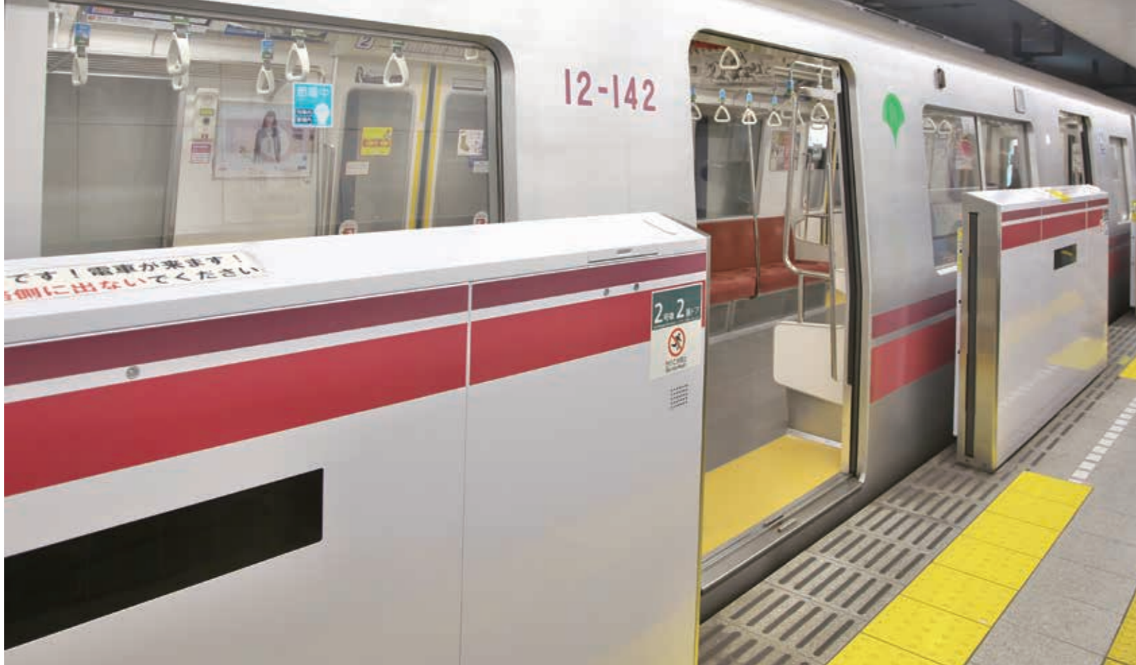
The Toei Oedo Line is working to ensure safety by installing platform doors and reducing the gap between the platform and the carriages.
