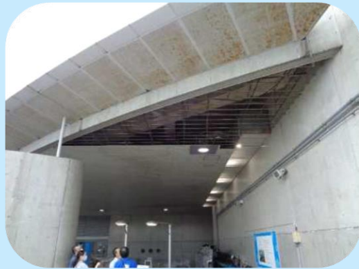
Corrosion of the ceiling bed *It has been repaired as of March 2023.
