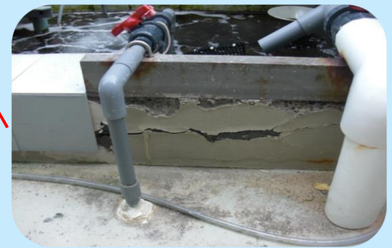
Deterioration of concrete (of the water tank)
