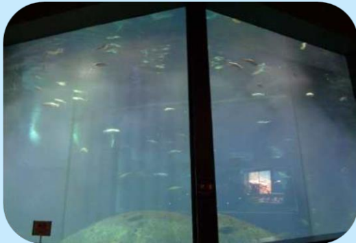
Cloudy acrylic and deterioration of glued parts
